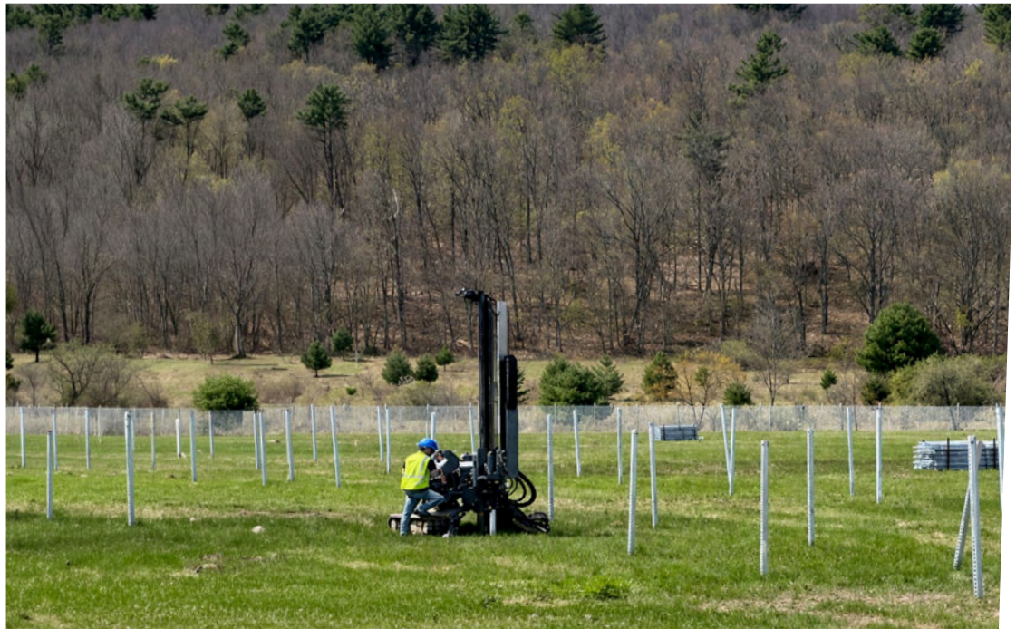
The 22 MW Payne Solar Project, built on the site of a former synthetic resin manufacturing facility in Bainbridge, NY.
