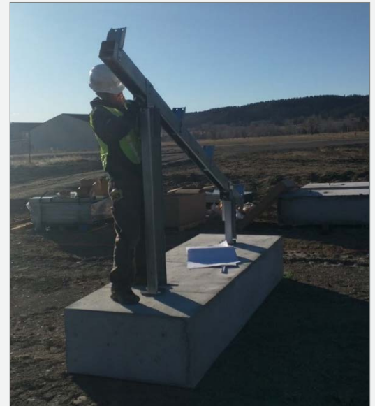
Above: The ballast blocks were formed on site with lifting anchors on them so that they could be moved easily, with standard construction equipment, in the future.
