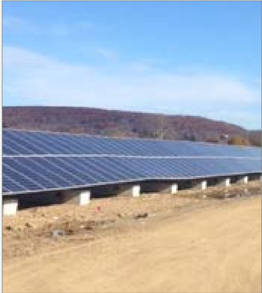
Above: Though the site was split into two locations, installation crews planned to unload all of the ballast blocks in one mobilization.
